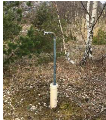
Fig. 25. Broken water tap near small lake.
