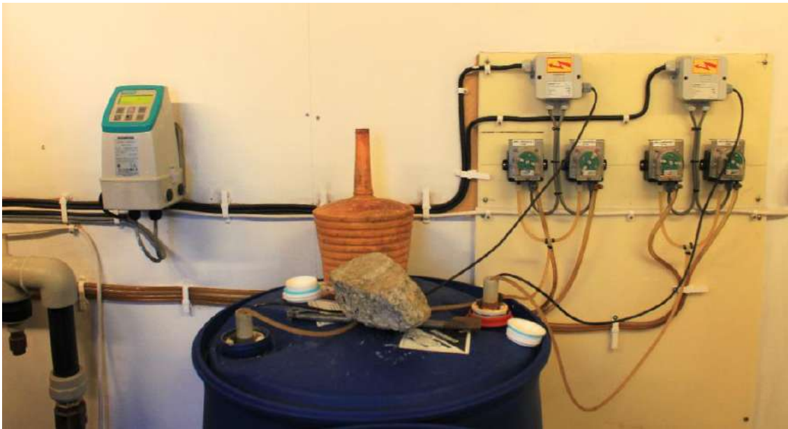
Fig. 20. The chemicals' dosage equipment at the central wastewater treatment system on Oaxen.
