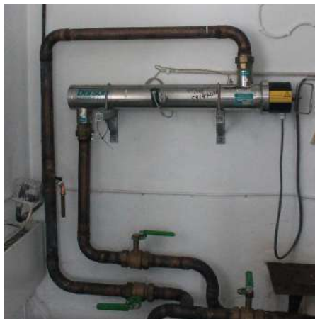
Fig. 16. UV-filter in the water distribution pumphouse.
