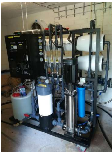
Figure13. The RoBUST 1000 Reverse Osmosis Desalination Plant. (Picture: Lotta Eriksson 2019.)
